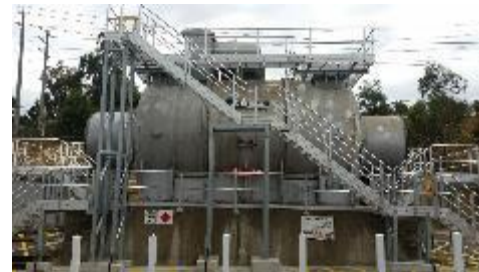
Example: Synchronous condenser/ Phaseshifter 125MVA. No shaft on left and right side. Source: Phasenschieber (Maschine) – Wikipedia
